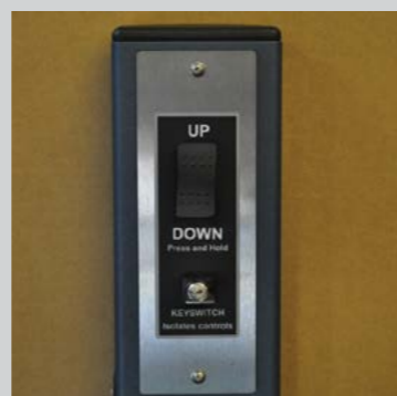
Key Switched Controls
