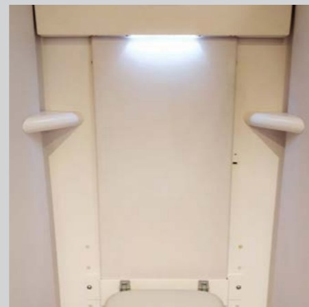
Battery Backup Powered Lights
